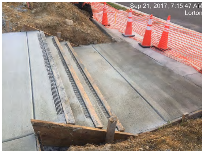
Steps are formed for the new platform entrance being added at Lorton.
