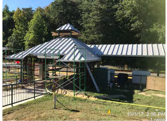
The Lorton Station Platform Extension project is also about improving the state of good repair of the existing station. The completed reroofing of the 25-year old shelter.
