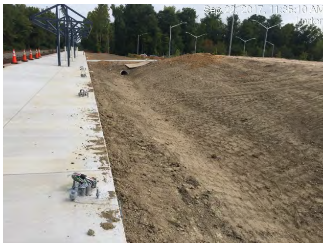
Initial grading of the drainage swale for the new platform extension at Lorton.
