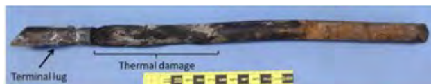
The NTSB’s photo shows thermal damage to an electrical power cable from a smoke incident at the Court House Metrorail Station
